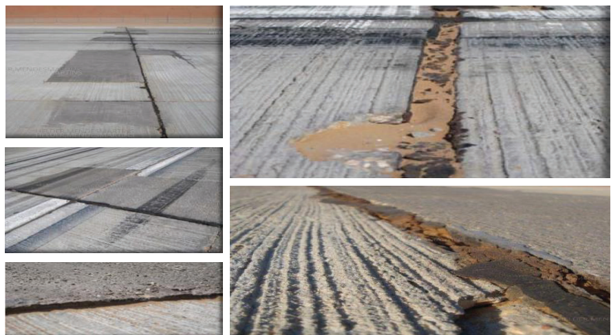
Figure 1: Deteriorated conditions of the old Shaybah Airport runway concrete pavement.
