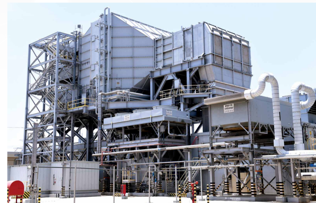
At Jazan, the refinery's vacuum residue is converted to syngas, which is used to power a 3.8 GW five-block combined cycle power plant producing electricity for both the refinery and the national grid, and generating steam for the refinery.
